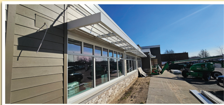
Construction at the Main Library at 407 William Floyd Parkway continues to progress month by month, with much of the exterior work finished including siding and windows.
