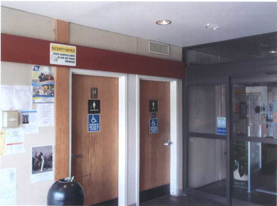
Photo 'H' Existing public Men and .Women toilet rooms in poor location and Not ADA Accessible
