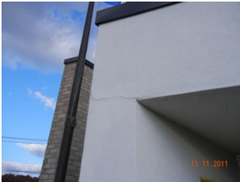
Closer view of the cracks in the finish. The finish should be exposed to determine the cause of the cracking.
