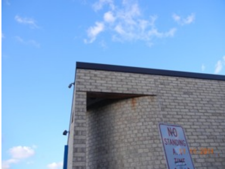
View of a steel lintel at the southwest corner of building. The steel is badly corroded.
