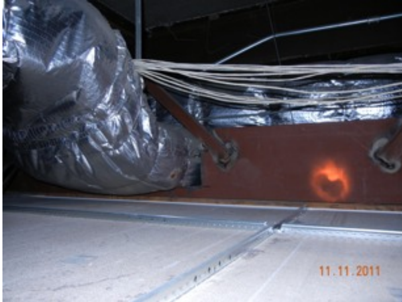
Another view of cut steel meant to support the movable partition below.
