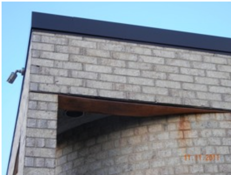
This is a closer look at the steel lintel. Note how the steel has pulled away from the masonry. It appears that this lintel has lost much of its strength. The bottom steel plate that we see could be pulled away from the steel frame above.
