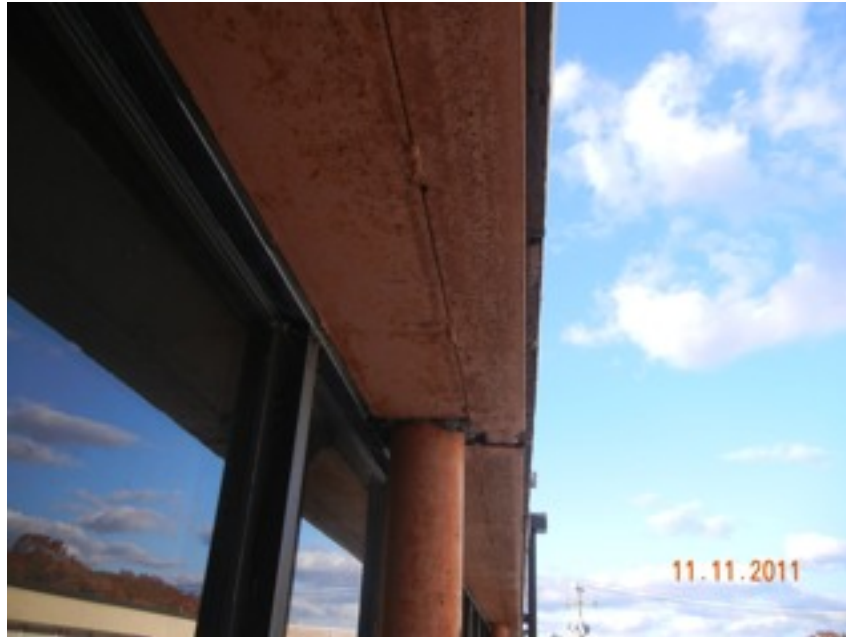
View of exterior steel lintels at clerestory windows in the original structure. The steel will require cleaning and painting.
