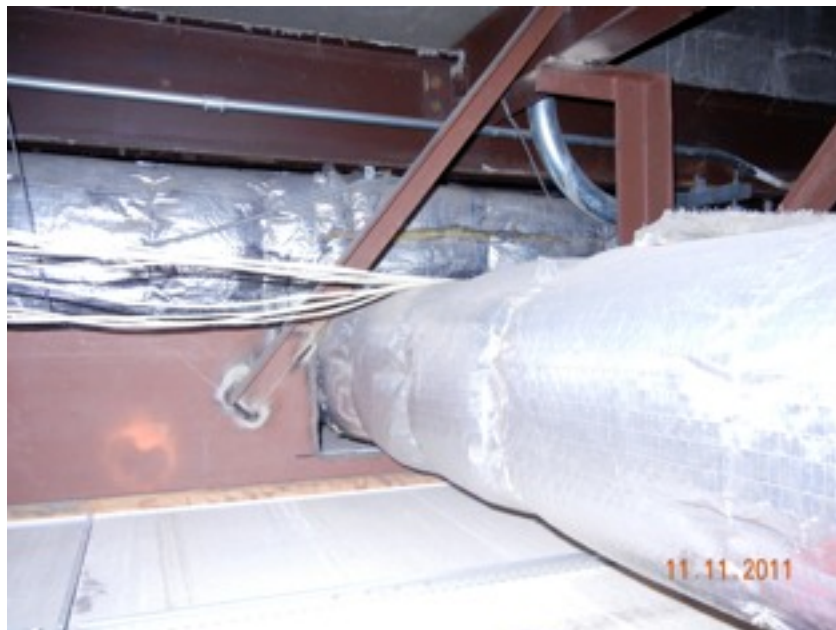
Another view of the cut steel hangers.
