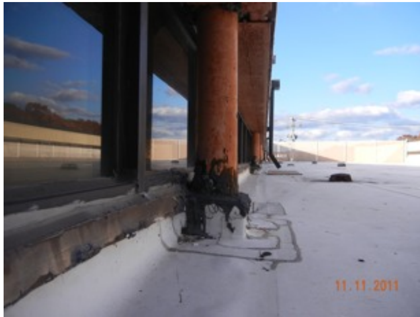
View of the lower sections of the same columns. We were able to note leaks below many of these columns. The columns should be cleaned, painted and reflashed if the leaks are active.
