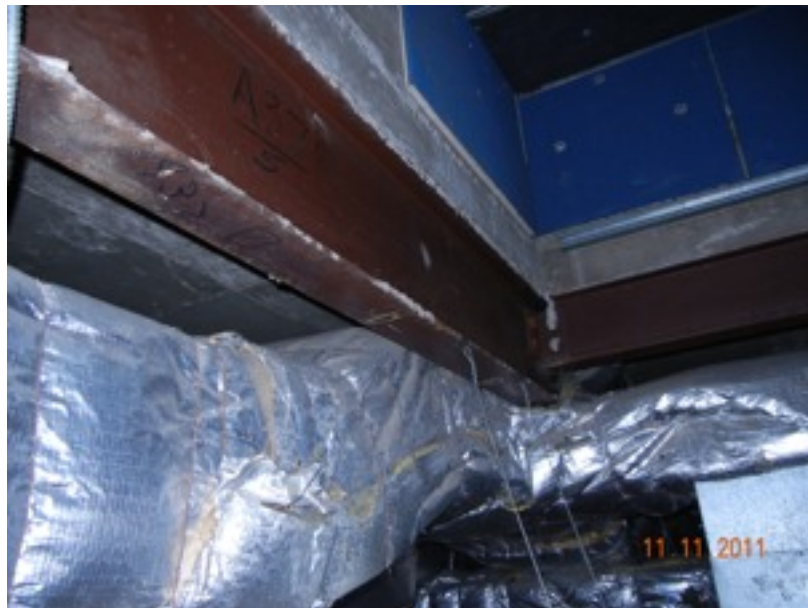
View of a steel framework that supports the roof top HVAC equipment. There are signs of minor water intrusion. The seals and flashing should be reviewed.
