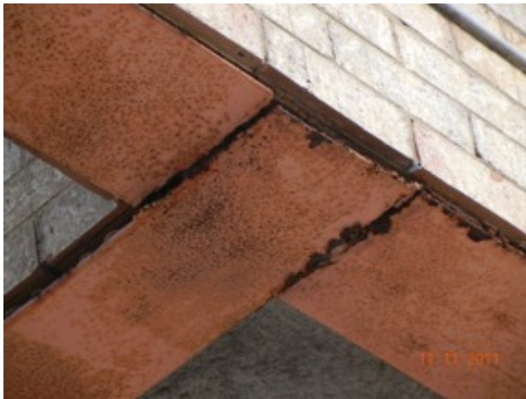
Closer view of the steel connection with the cantilevered girder. Note that much of the corrosion is above the steel, behind the masonry. The masonry will need to be removed to expose all of the steel.
