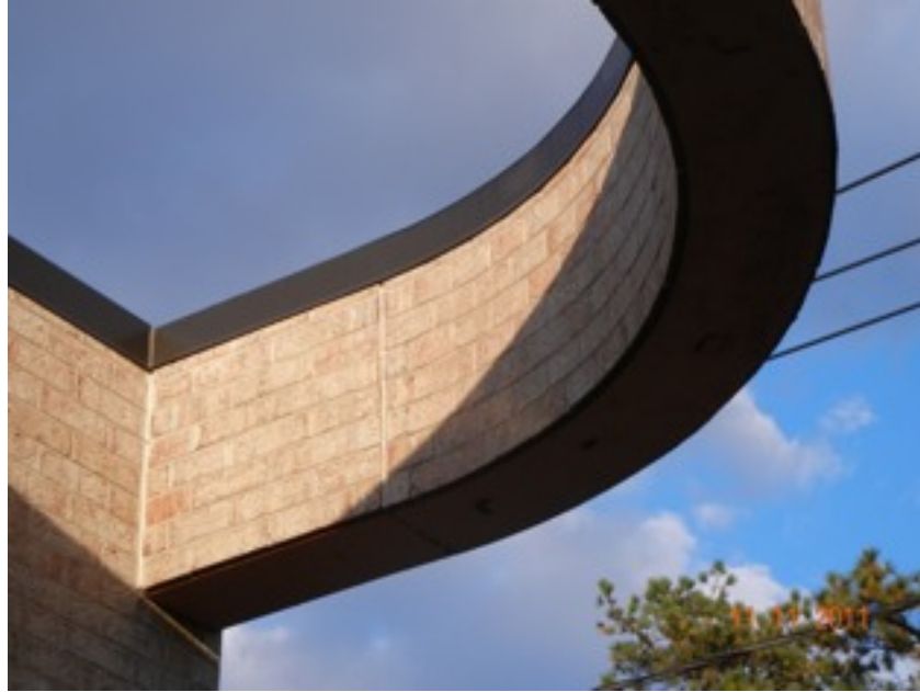
View of a curved header at the rear of the building. There is corrosion of the steel along the length of the header.
