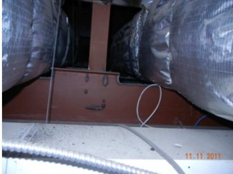
View of steel hangers in the newer portion of the building. The cut steel is not of concern. It appears that the hangers are only meant to support the HVAC ducting and a movable wall partition below.
