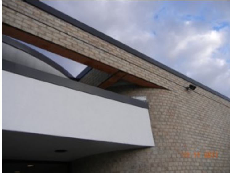
View of the steel lintel over the main entry. In this case there is a steel girder cantilevered out from the main building. Much of the steel is corroded.
