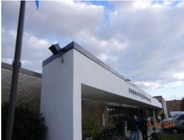
View of the front awning. I was able to note cracks at the intersection of the awning and supporting end wall.
