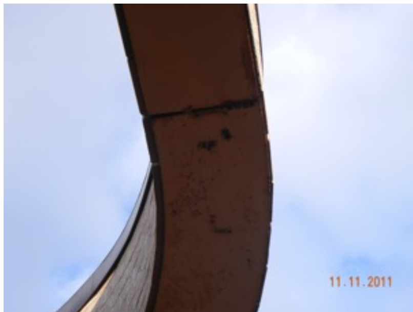
Closer view of the curved header. There is a steel connection along the length of the lintel. The masonry will need to be removed to inspect, clean and paint the steel.
